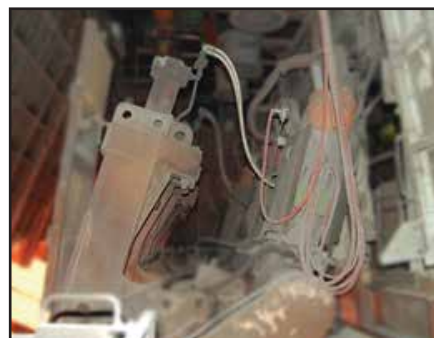
Temperature Monitoring In A Continuous Casting Plant
