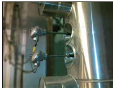
Temperature Sensor For Steam Pipelines In A Chemical Plant
