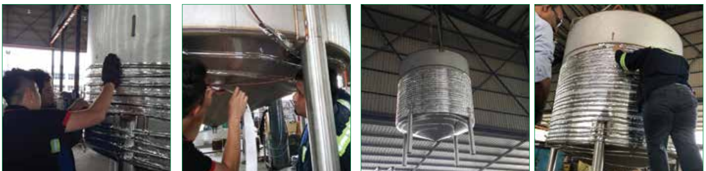
Design, Commissioning and Installation of Heat Tracing Cable for Palm Oil Industry
